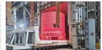
• Heat Treatment Furnace (Max. 300t, 11.2M (W) x 6.5M(H) x 20.2M(L))
